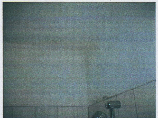
Schimmel in badkamer
